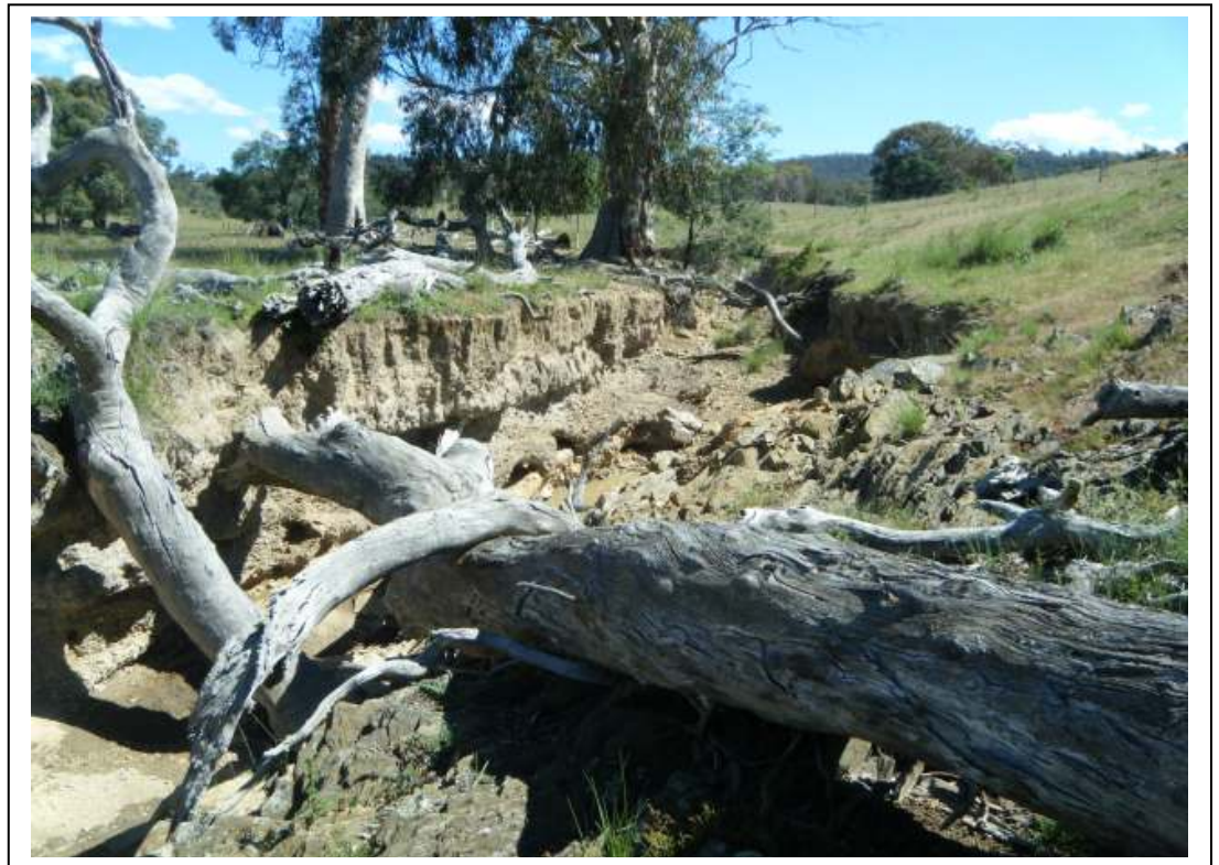
Lower section of the erosion area
